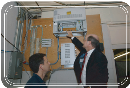
Greg McConnell of Louisiana Office Supply (left) and Richard Peak of Preferred Telephone designed a Toshiba Strata CIX system with battery backup so the system stays live even with power surges and outages.
